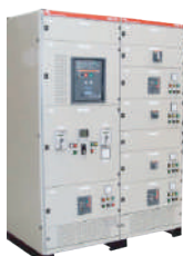
Main Low Voltage Switchboards
